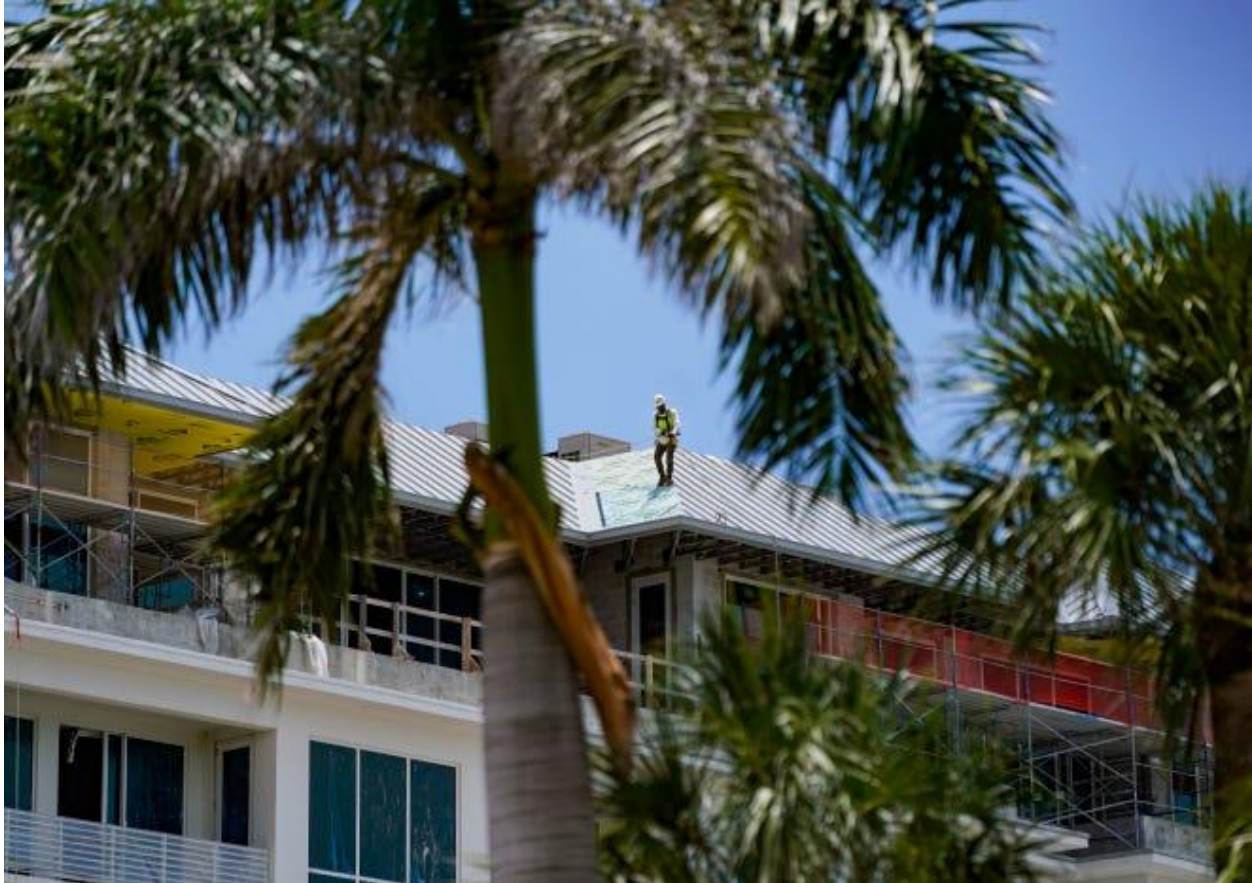
Construction continues near the Naples Beach Club on Gulf Shore Boulevard North in Naples, Fla., on Thursday, July 10, 2025. Jonah Hinebaugh/Naples Daily News/USA Today Network-Florida
