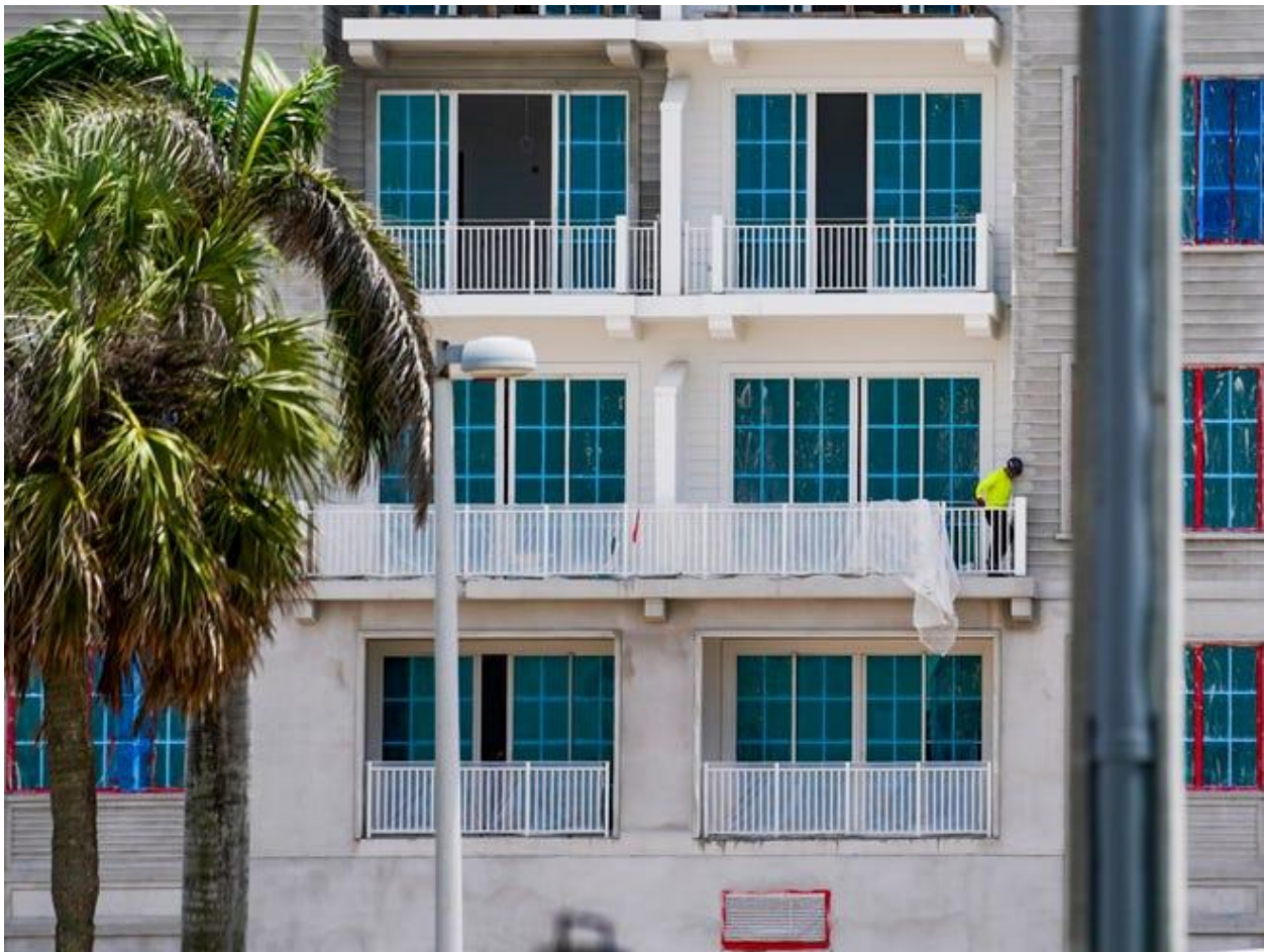
Construction continues near the Naples Beach Club on Gulf Shore Boulevard North in Naples, Fla., on Thursday, July 10, 2025. Jonah Hinebaugh/Naples Daily News/USA Today Network-Florida
