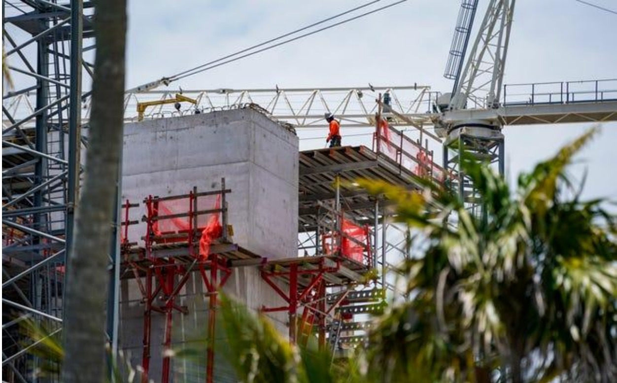
Construction continues at Rosewood Residences on Gulf Shore Boulevard North in Naples, Fla., on Thursday, July 10, 2025. Jonah Hinebaugh/Naples Daily News/USA Today Network-Florida
