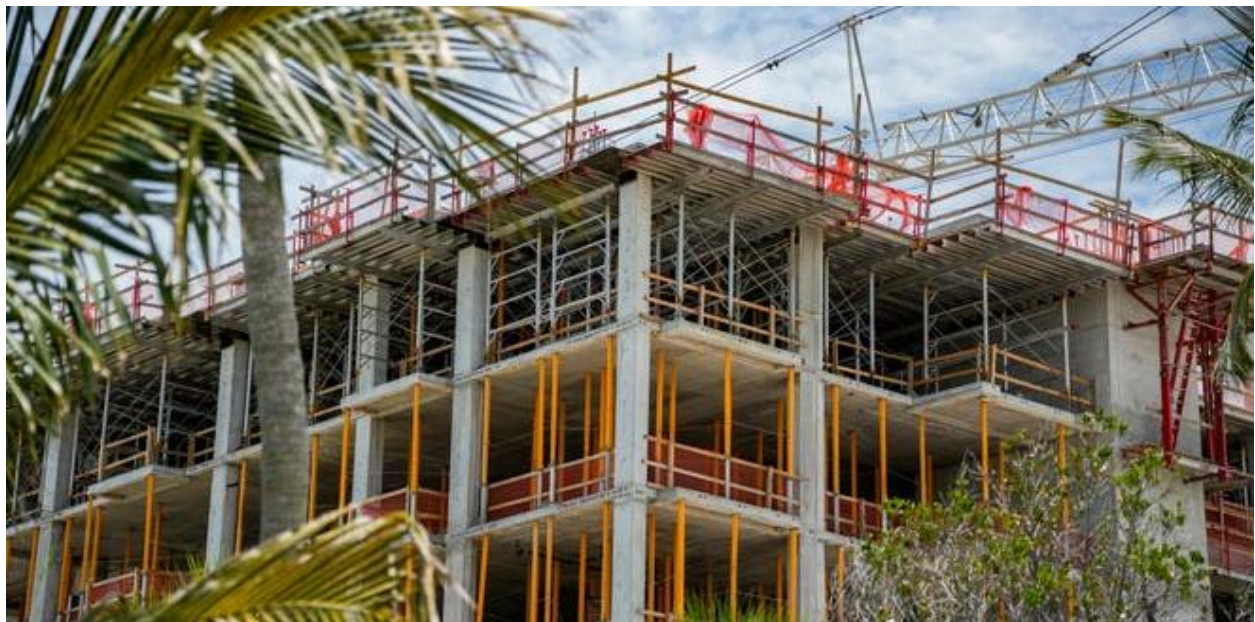
Construction continues near the Naples Beach Club on Gulf Shore Boulevard North in Naples, Fla., on Thursday, July 10, 2025. Jonah Hinebaugh/Naples Daily News/USA Today Network-Florida
