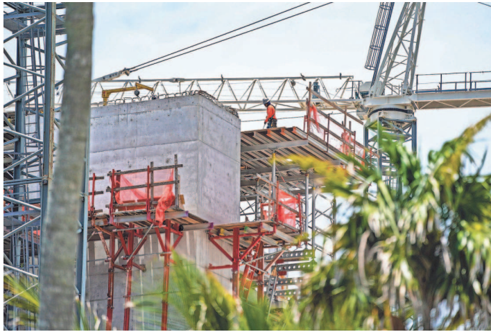
Construction continues at Rosewood Residences on Gulf Shore Boulevard North in Naples on July 10.
