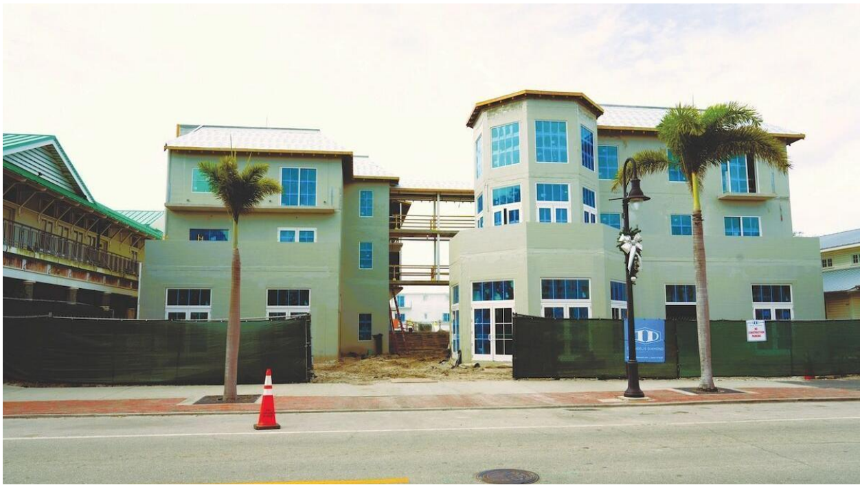
The 109-room Old Naples Hotel is being built on the site of the former Plaza on Third Street, bordered by Third Street South, Broad Avenue and Gordon Drive in downtown Naples. Tim Aten
