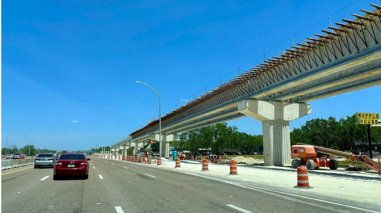
Florida Department of Transportation began construction in 2025 on a flyover at Collier Boulevard and Davis Boulevard in East Naples as part of the Interstate 75 interchange project. Tim Aten
