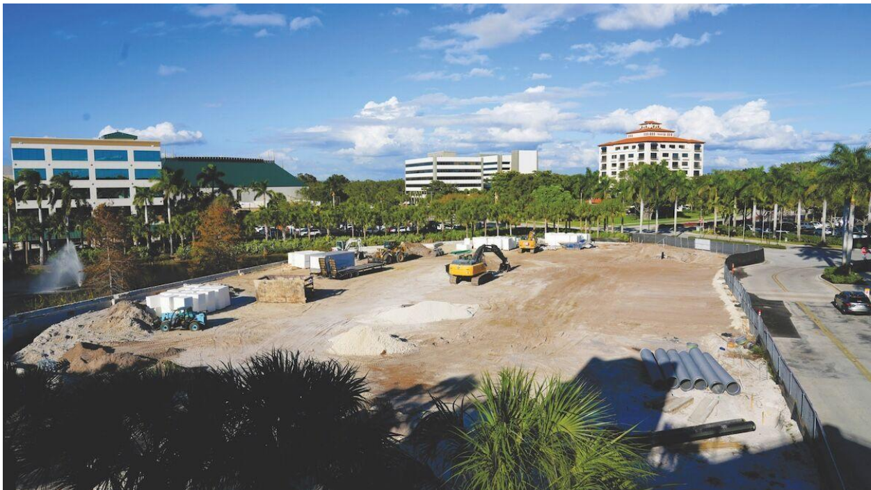
DeAngelis Diamond recently began construction of Restoration Hardware Naples with a luxurious RH restaurant on the footprint of the former Nordstroms department store at Waterside Shops. Tim Aten
